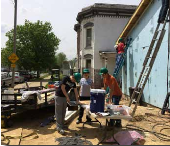
Airmen from the 139th Civil Engineer Squadron, volunteer to help build a house for Habitat for Humanity, May 17, 2014. (U.S. Air National Guard photo by: Lt. Col. Grace Link)
